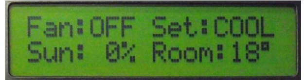
Main screen in a solar Air Heater system
