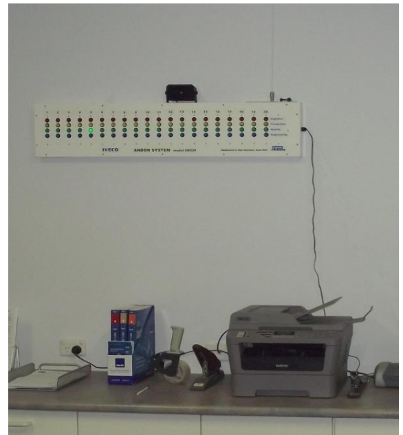
The wall mounted Central Panel
