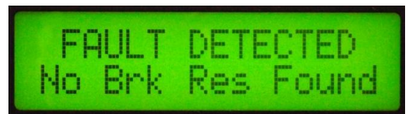
Display showing brake resistor fault
